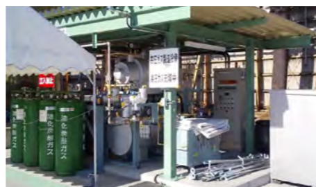
Exterior of the CO 2 liquefaction system
